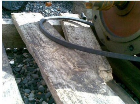
X Broken planks
