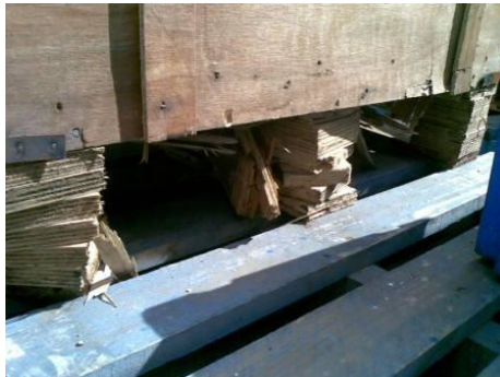
X Poor wood structure
